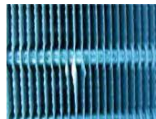
Cooling coil fins 60 day after UVC
