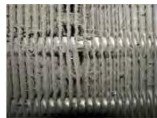
Cooling coil fins before UVC
